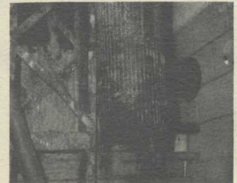
The lower portion of the well screen showing the place where the lower 3 ft. had rusted off.
