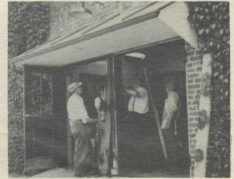
Bill Sallow, Harry Clark, Erv Braatz and George Currier, of the Maintenance Department, remove center post of door to allow clearance for the well rig.
